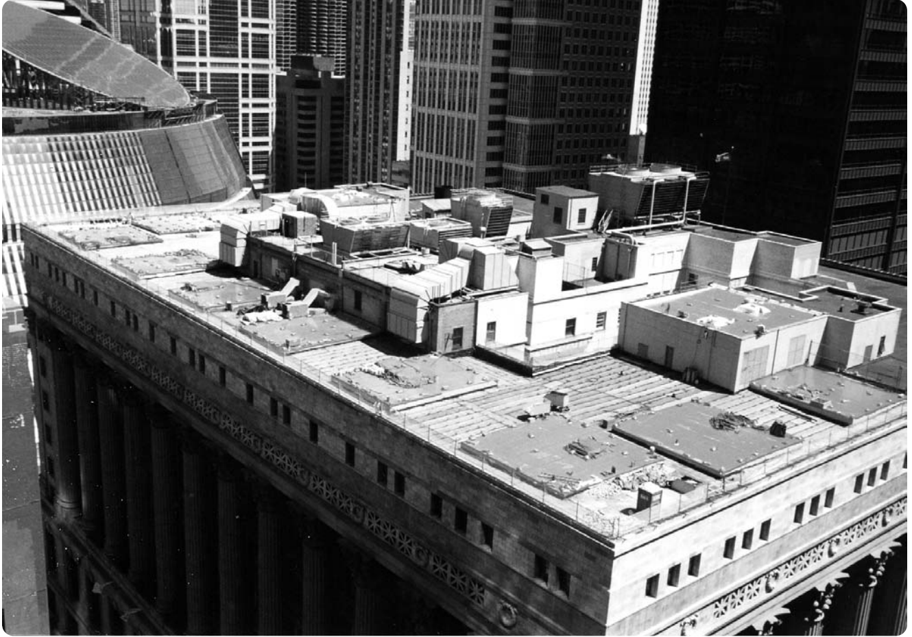
The rooftop garden at City Hall under construction, Chicago. (MARK FARINA, DEPARTMENT OF ENVIRONMENT, CITY OF CHICAGO, 2000)
